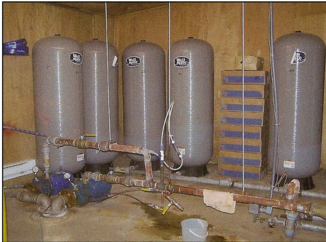
Expansion Tanks (bladder tanks)
