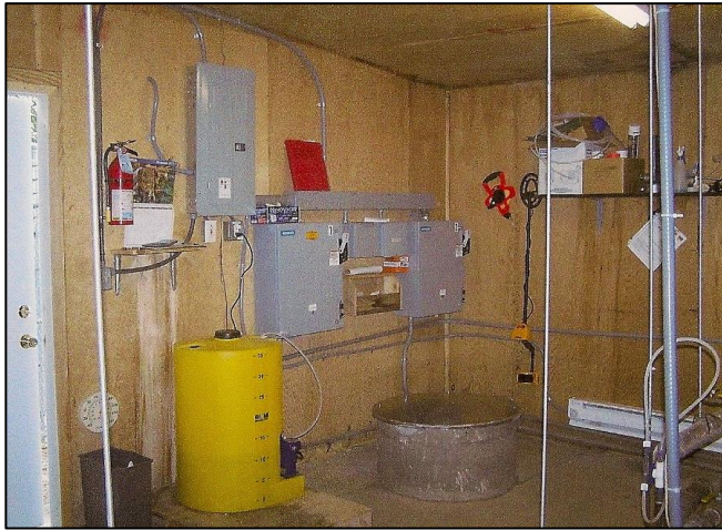
Interior south wall of pump house: chlorination tank, panels, and cistern tank.
