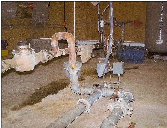
Main water line to system, expansion tank connecting lines, water pumps.
