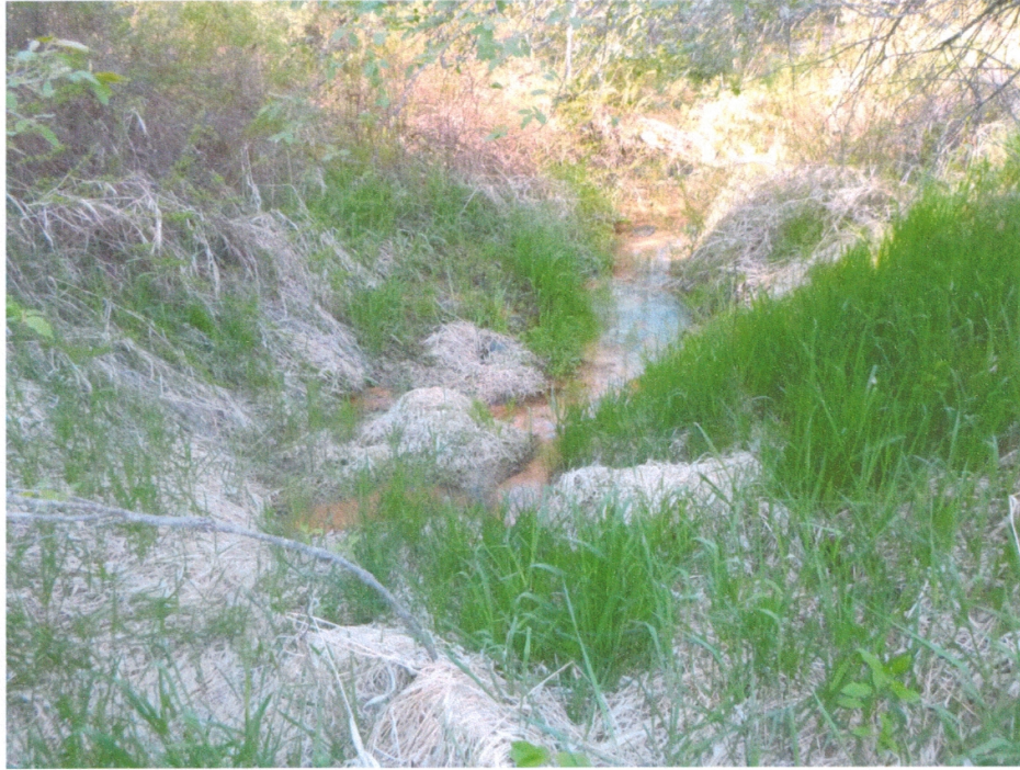
Photo 15: Seepage near the left abutment on South Dam
