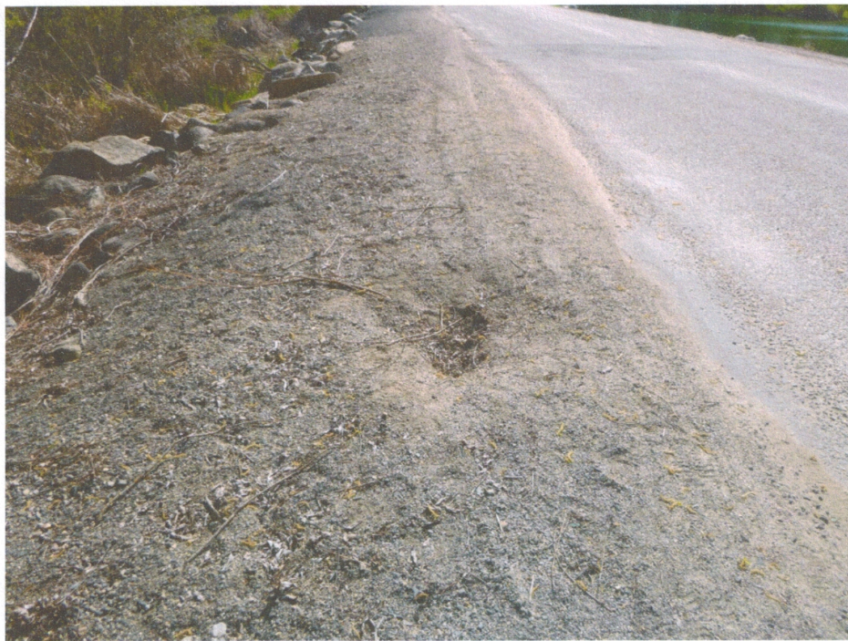
Photo 16: Slumping area near the left abutment on North Dam
